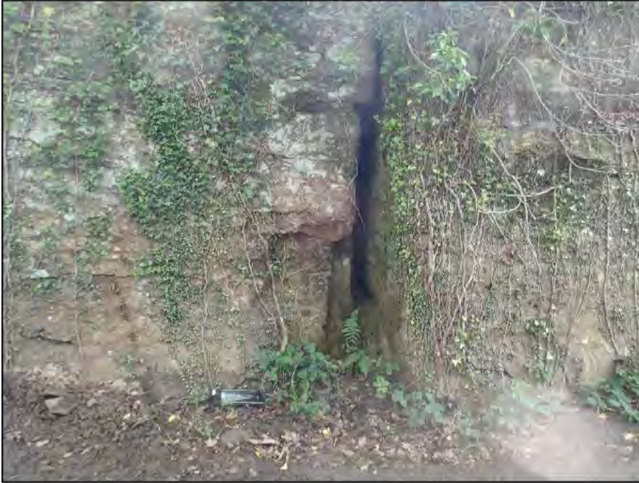
Plate 5: Bedding dipping from left to right (20/185) the rock face is formed by joint set 84/274 and the dilated joint set is formed by 74/018.
