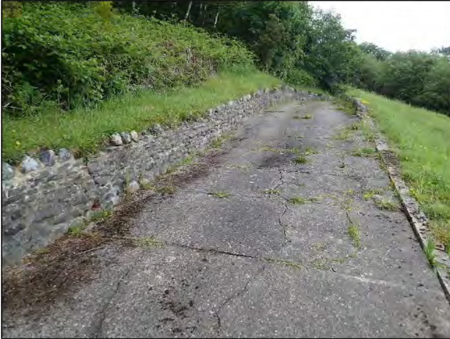
Plate 8: Distress evident in the upper part of the cemetery.
