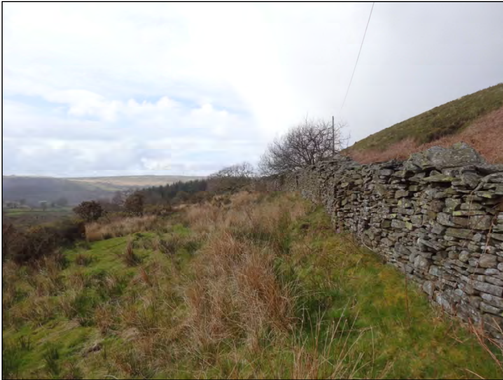
Plate 7: View along rear of landslide, note adit (M3) in the right of the photo. Note no drainage ditch. Photo taken looking west.
