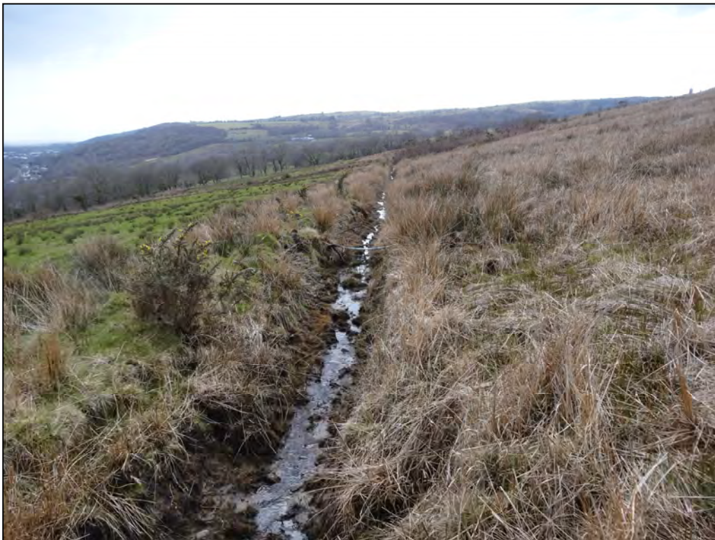
Plate 12: Photograph of ditch running along the southern margins of the landslide, looking west. Note difference in grass either side of ditch.
