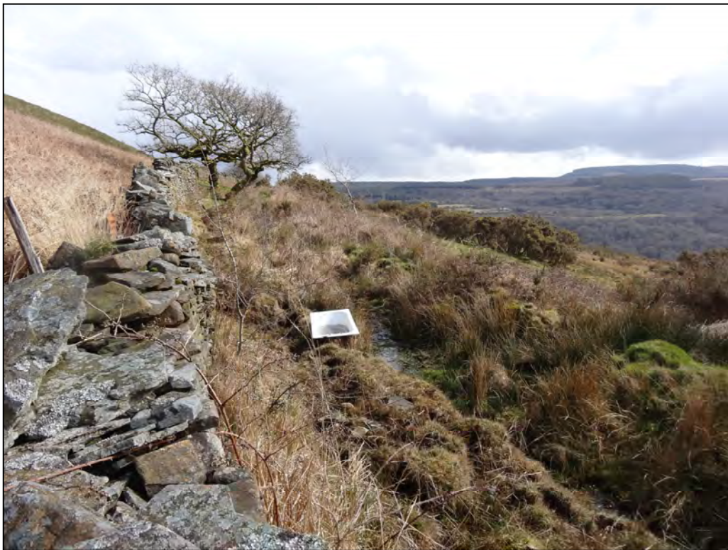
Plate 18: Photo looking east along ditch at the rear of the landslide.
