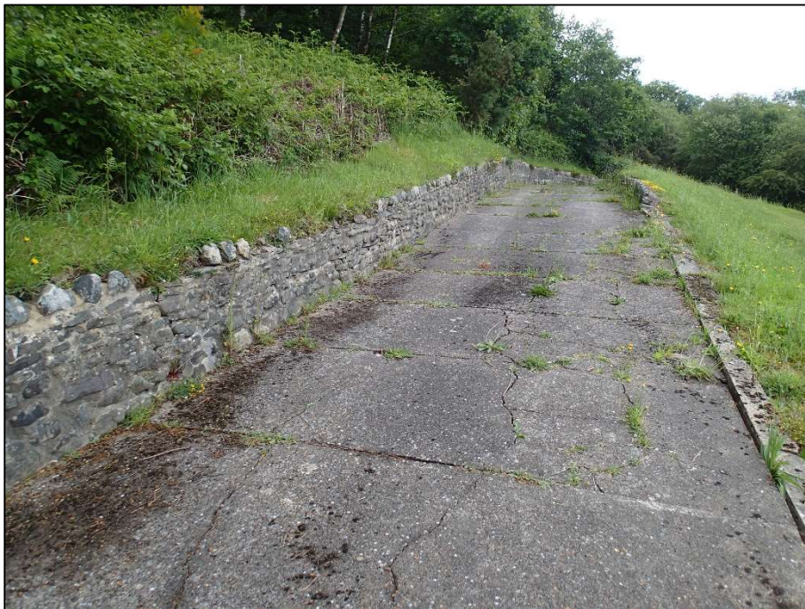
Plate 9: Distress evident in the upper part of the cemetery.
